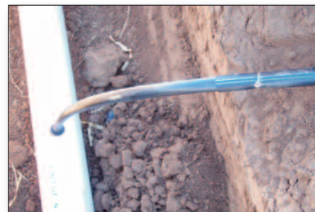
Jordan shanked in his 7/8 inch, Toro Aqua-Traxx drip tape 12-15 inches deep on 80 inch centers. The emitters were 16 inches apart, and the flow rate .17 gpm per 100 feet, resulting in an application rate of .025 inches per hour. Tape laterals were connected to buried PVC pipe.
